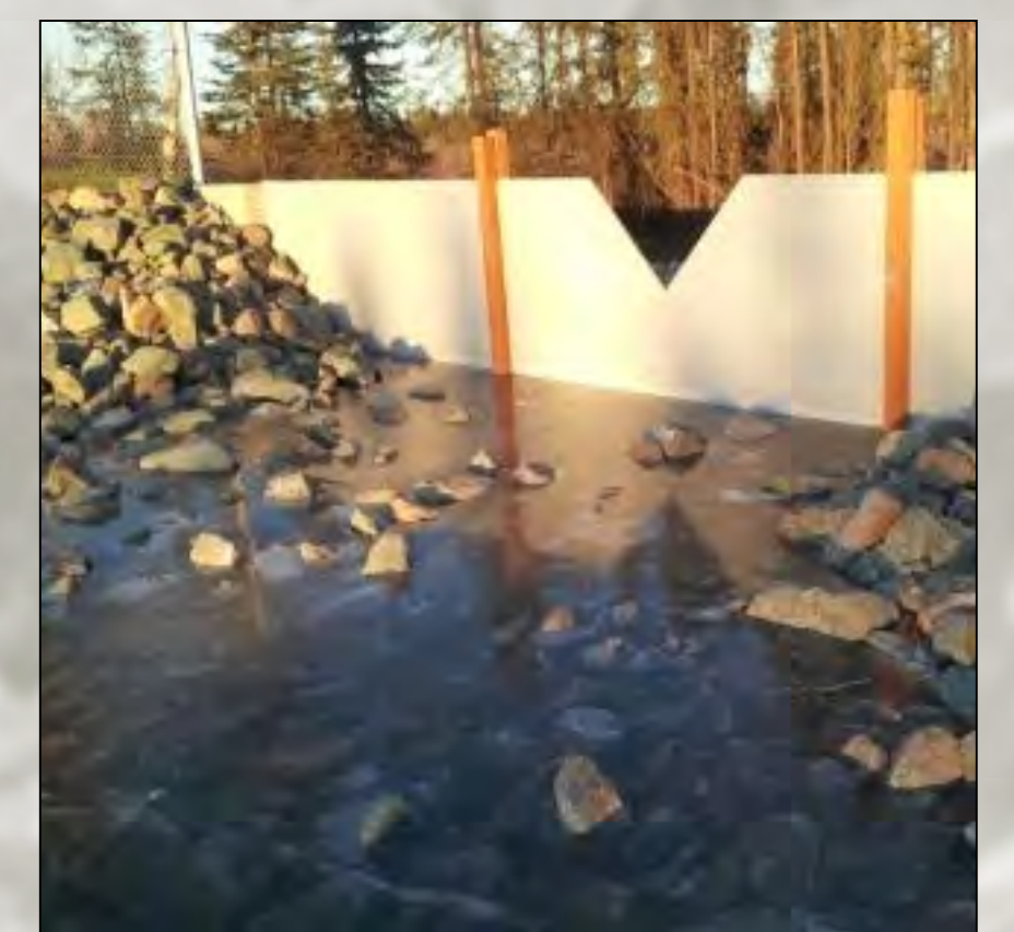
Dry Detention Volume Draining/ice obstruction
